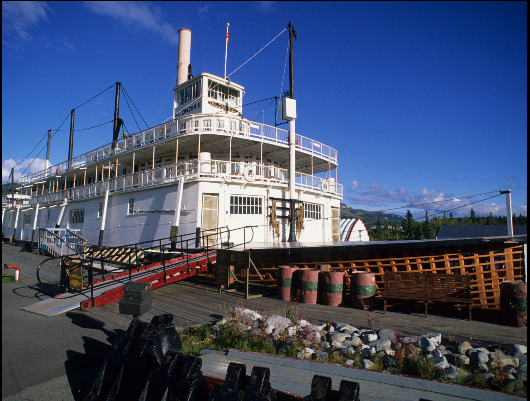
76 The Klondike paddle wheeler in Whitehorse, Yukon while undergoing reconstruction. This is one of two remaining sternwheelers in the Yukon. During the gold rush on 1898, 100's of similar boats traveled from the Whitehorse to the gold fields of Dawson.
